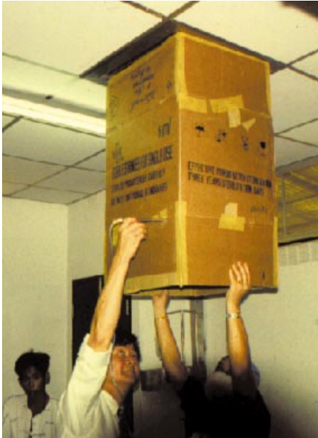
Using a carton box and flow velometer to monitor air flow in TB patient isolation room with mechanical ventilation system, Chiang Rai Hospital, Chiang Rai, Thailand
